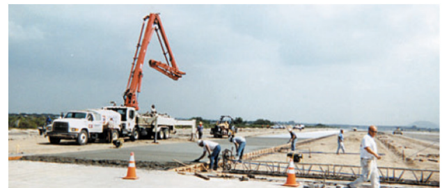
Point Mugu Naval Air Station required a 565-foot long, non-jointed pour of 30% Class F fly ash concrete.
